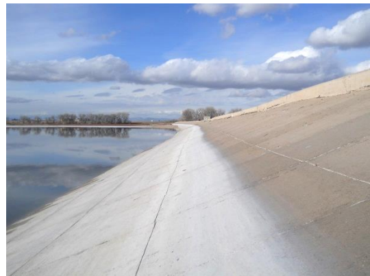
"Bathtub ring" of calcium deposit at Barr Lake
